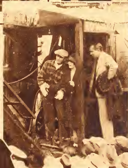
1927—With Doug looking on, Mary operates steam shovel that breaks ground for new Los Angeles theatre, which later opens with "My Best Girl"
